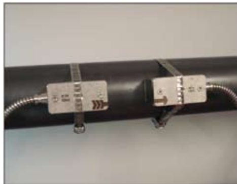
Transducers mounted using strap and clamps
