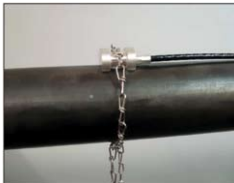
PT100 sensor fixed to pipe
